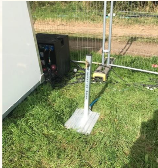
Drinking water pipe
